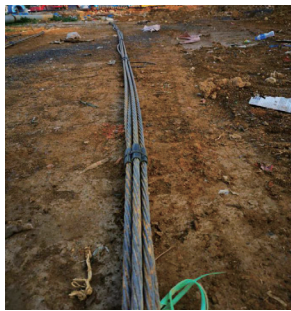
> 图6 复合锚杆杆筋制安 > Fig.6 Fabrication and installation rebar of composite anchor
